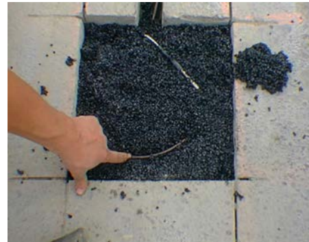
Figure AK-3. Top sensor on a wire lead.
